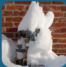
METER WITHOUT SNOW SHELTER
